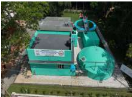
360 KLD STP at General Hospital, Thrissur
