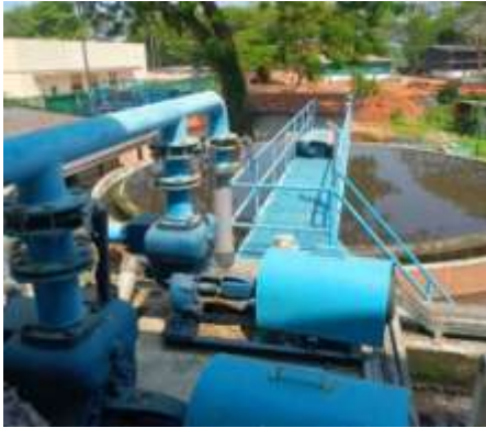
500 KLD STP at Kozhikode medical College
