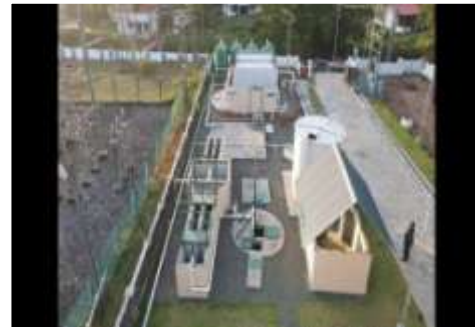
1 MLD CSTP at Padanappalam, Kannur
