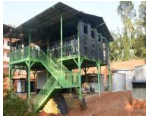
1 MLD STP at Kozhikode medical College
